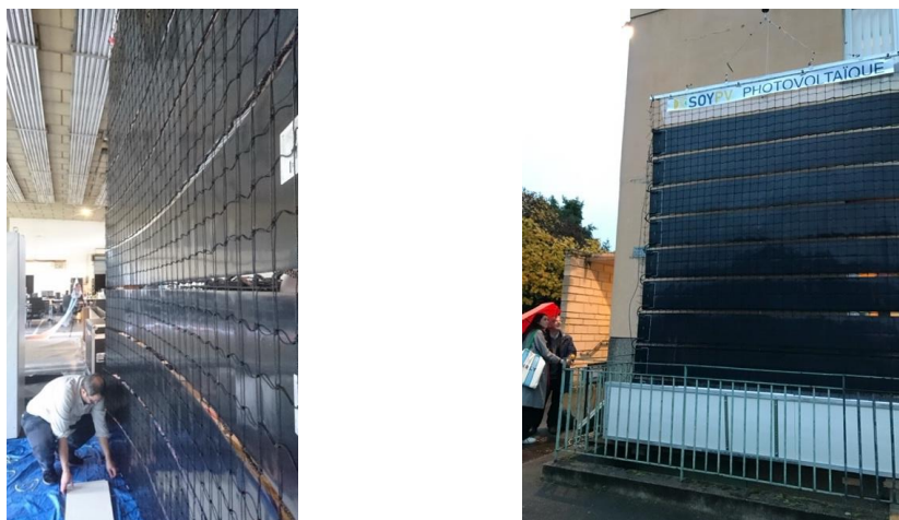
Fig.1 : On the left, photovoltaic veil made by SOYPV in the CNRS-UPS platform at the University Paris Saclay; on the right, deployment of the veil on the facade of a building in Aulnay-sous-Bois
